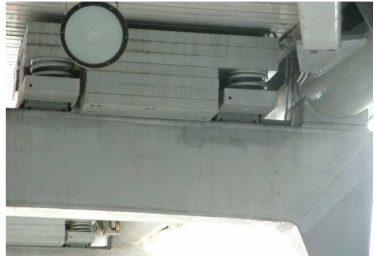
London Millennium Bridge Mass Dampener (Floats on Springs)
